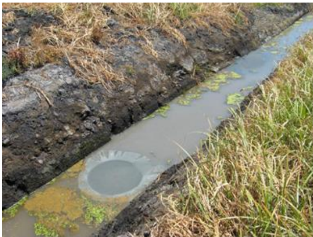
Figure 6. Active boil on Jones Tract observed in 2011. Photo credit: Gerald Bawden
